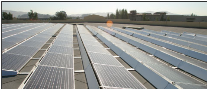
Tilt Angle Flat Mounted Roof System (2 50KW Systems Hopewell Twp., 2006/07; 8KW MSOTF 2006)
