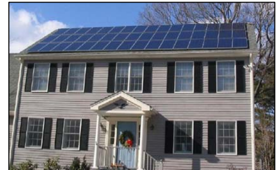
Slope Mounted PV (8KW Holmes Residence, Manchester, NJ, 2007)
